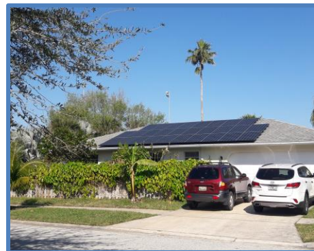
Figure 15. Resident David Vigliotti's home solar array now provides his family with almost zero electric utility expenses.
