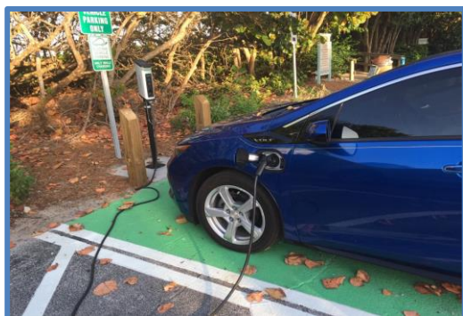
Figure 14. Pelican Beach Park electric vehicle charging station.
